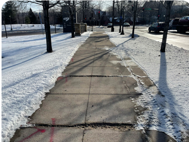
Poor sidewalk conditions
